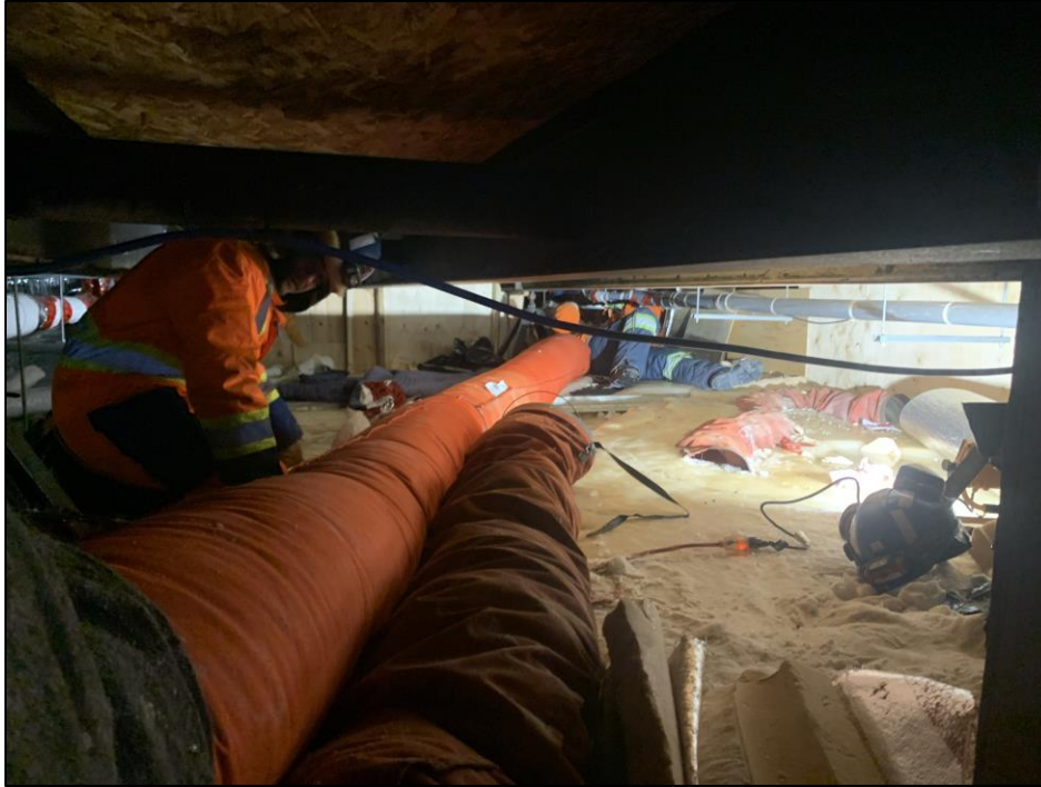
Photos 2: Greywater spill location, underneath the kitchen building.
