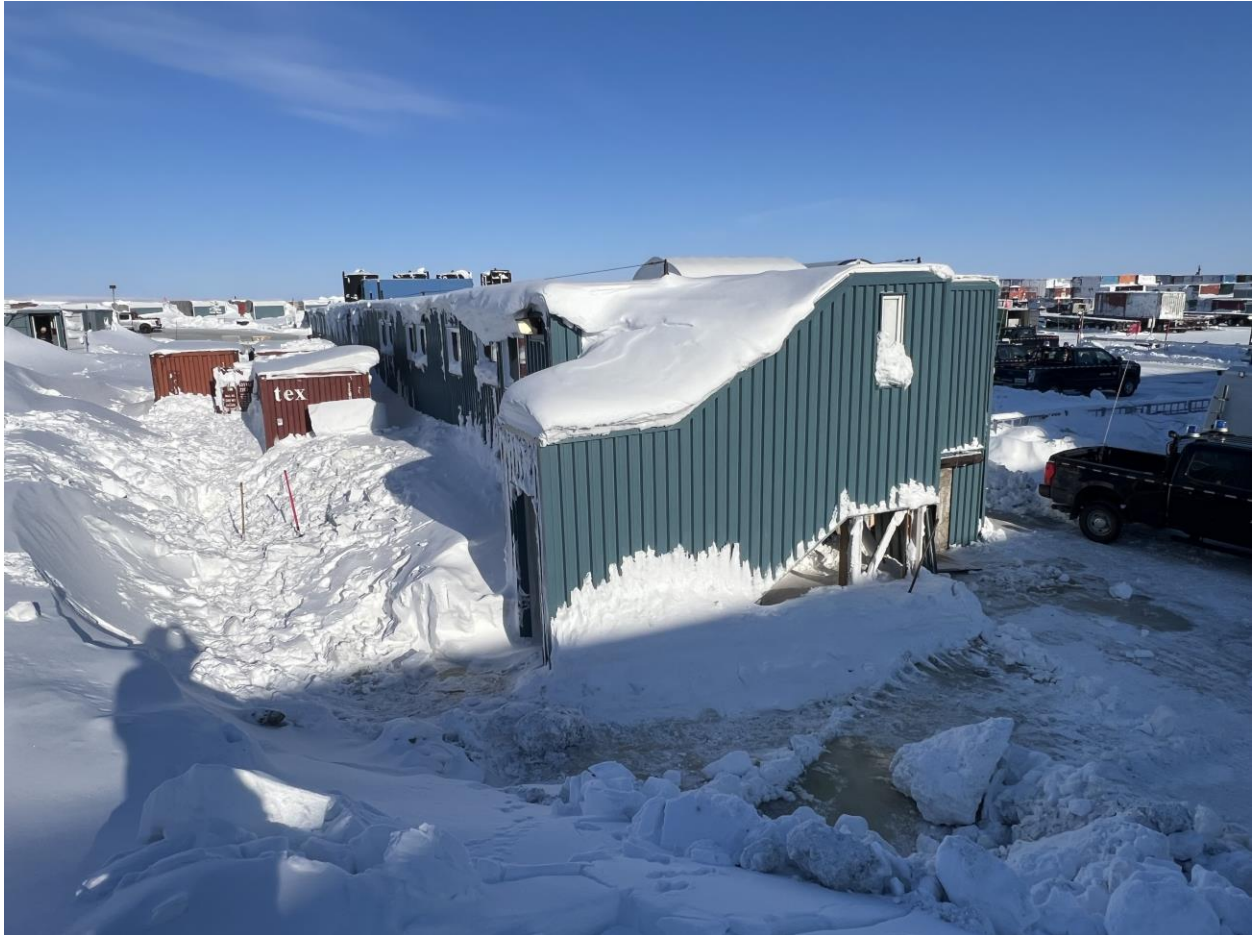
Photo 1: Sewage spill location
