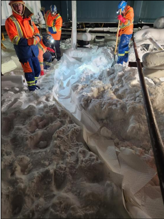
Photos 1: Spill location
