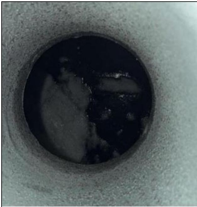
Photo 2: Paraffin in diesel tank from summer fuel being left in tank too late into winter.
