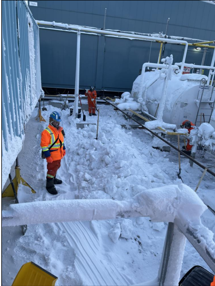
Photo 3: Spill location during remediation
