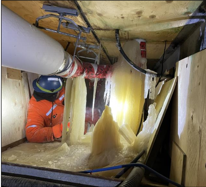
Photos 1: Greywater spill location, underneath the kitchen building.
