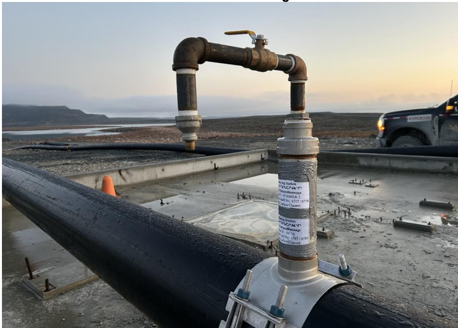
Photo 1. FDP Vault Attenuation Pond Discharge Meadowbank
