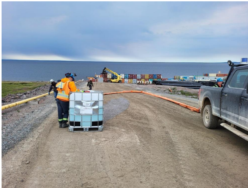
Utilizing spill booms and spill pads to control the flow.
