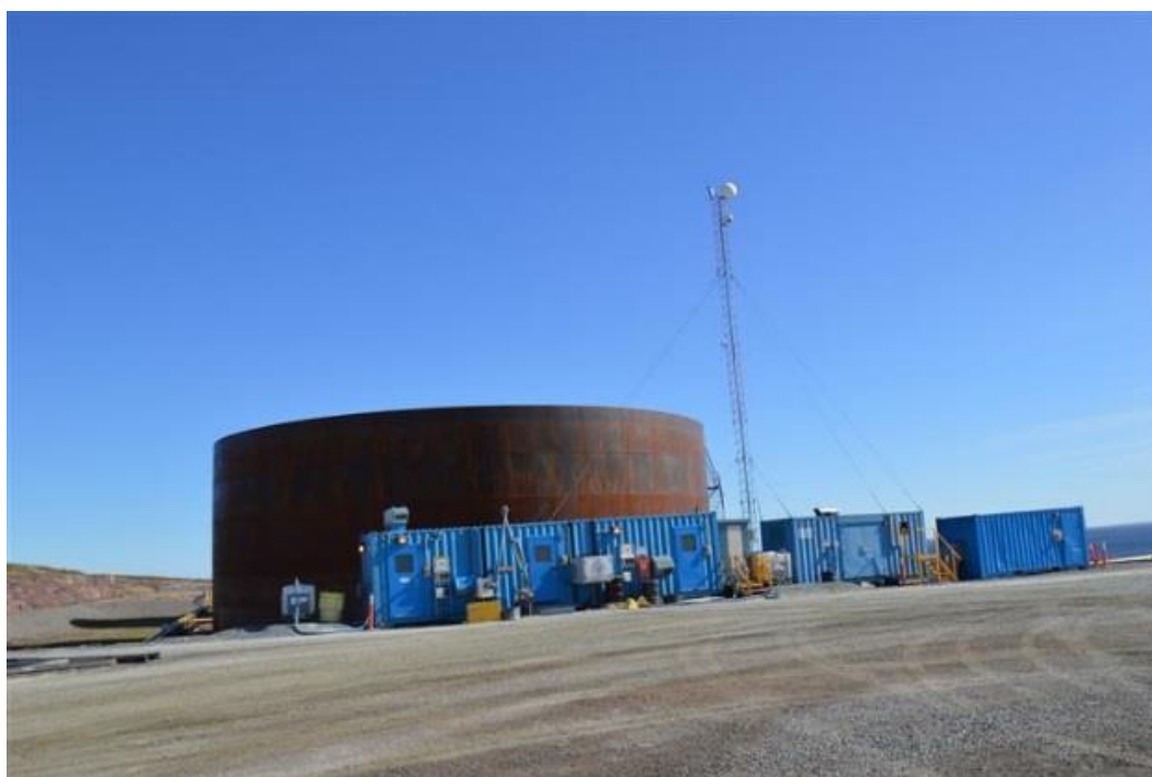
Photo 4: Agnico Eagle Ltd.'s Refueling Station – general view
